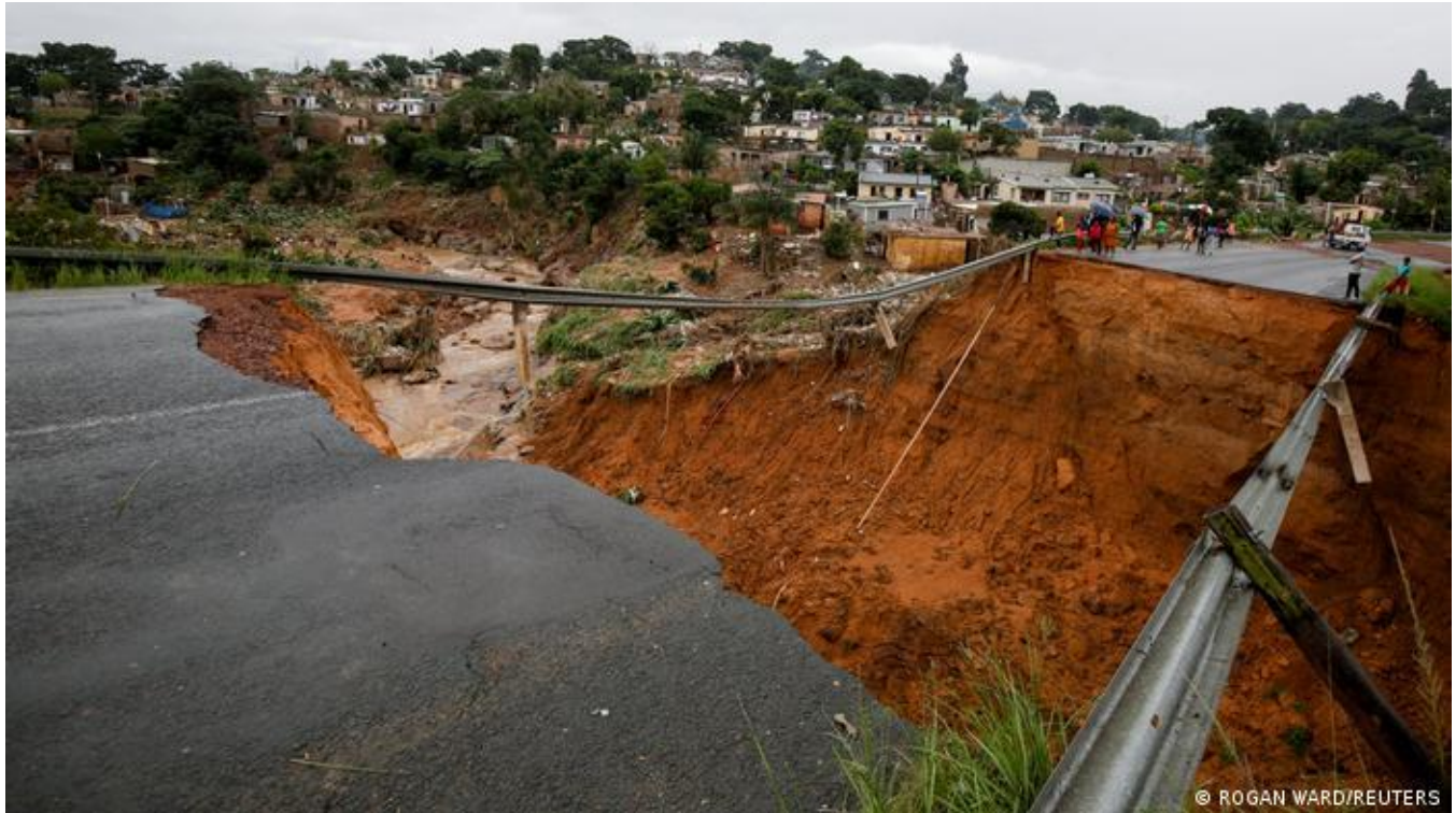
Massive damage to infrastructure
